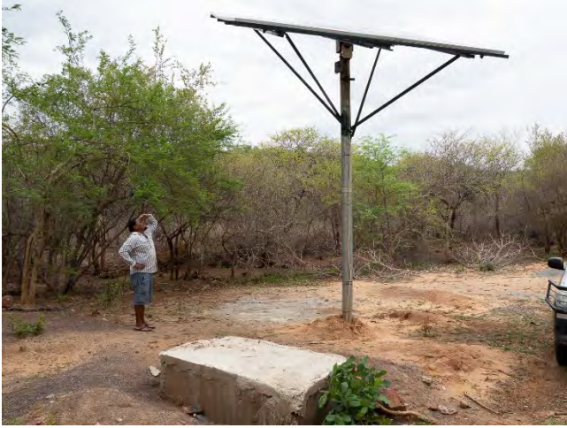
The new borehole – the pump is enclosed in very thick concrete. Security cameras are being installed.
